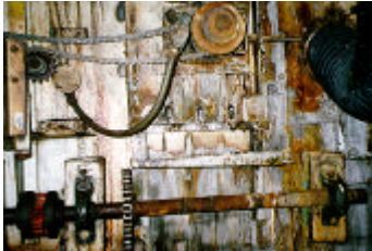
Figure 1. Corrosion of machinery & parts
