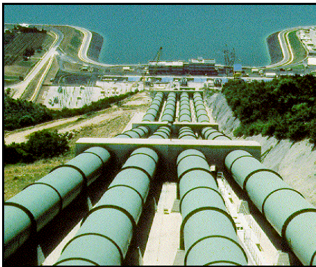
Figure 1: Photo of a typical penstock system
