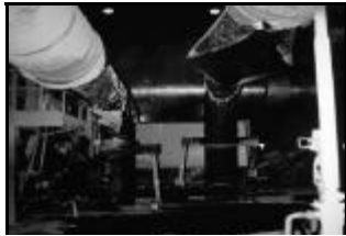
Figure 1: A seam-weld failure
