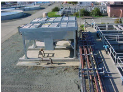
Engine Cooling Water Piping & Radiators
