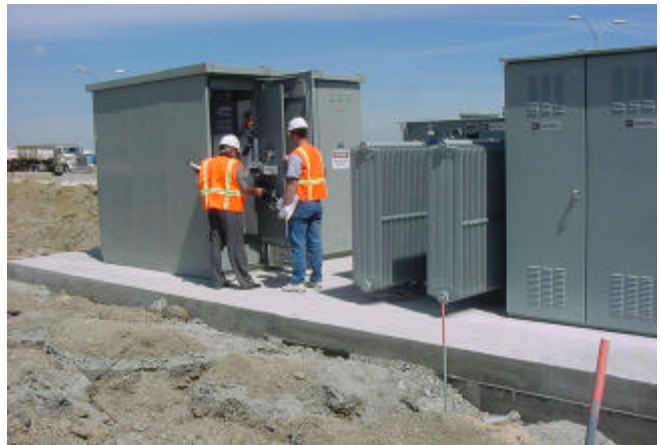
Generator Substation Showing Switchgear, Transformer, & MCC
