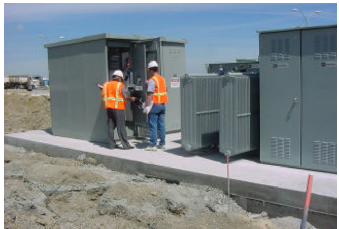
Generator Substation Showing Switchgear, Transformer, & MCC
