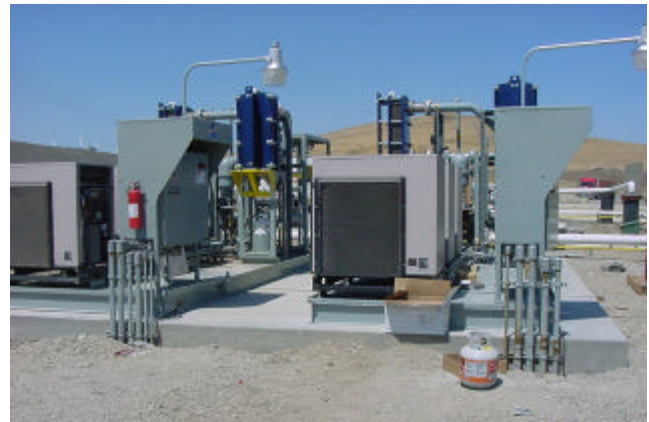
Landfill Gas Conditioning Units
