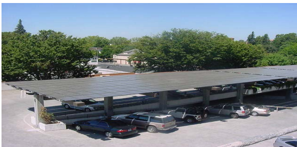
Parking Structure Roof with Fixed PV Array providing Power and Shade
