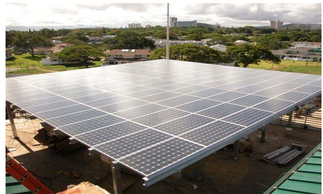
Roof Canopy Fixed PV Array System providing Power and Shade (Hawaii)
