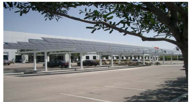
Tracking System providing Power and Shade
